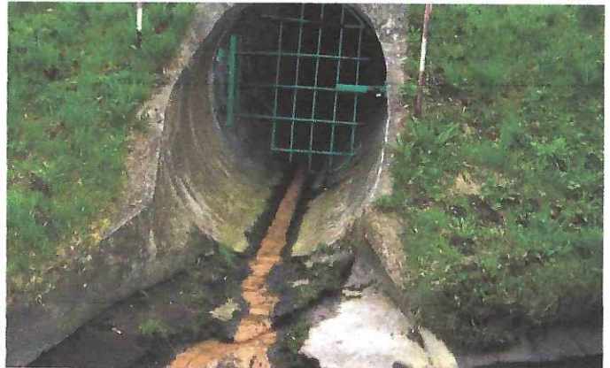
Potential illicit discharge flowing out of a concrete outfall. Confirming an illicit discharge may require sampling or other investigative methods to determine the pollutant and responsible party.
